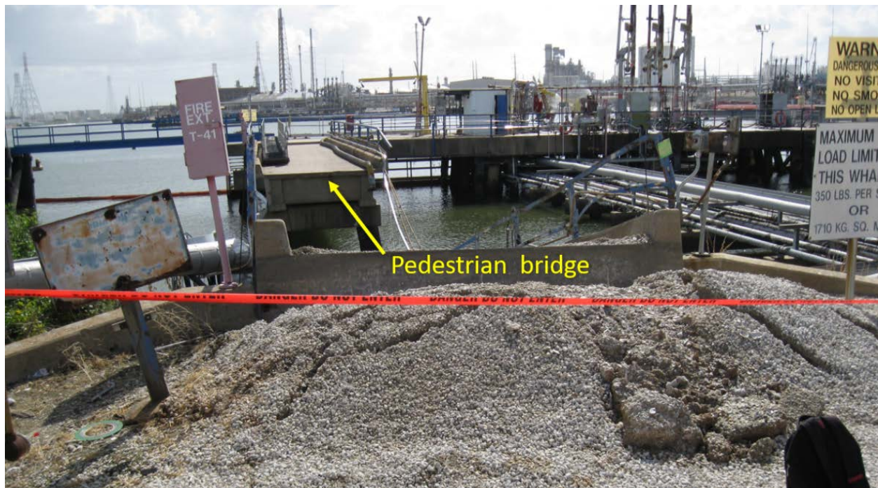
TPC facility on Houston Ship Channel. The impact pushed the pedestrian bridge off its support, crushing conduit below. (Photo by Coast Guard)
