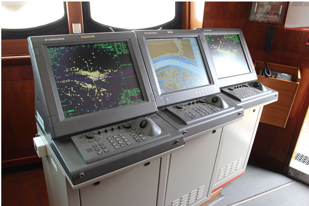
Figure 2 – Radar and ECDIS displays on a merchant ship bridge.
